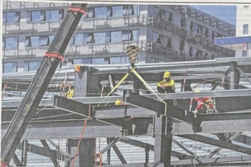
WORKING ON A HOLIDAY Construction crews assemble a building frame along Bioko Boulevard in Pasay City as the country marked Labor Day on May 1, 2026.
